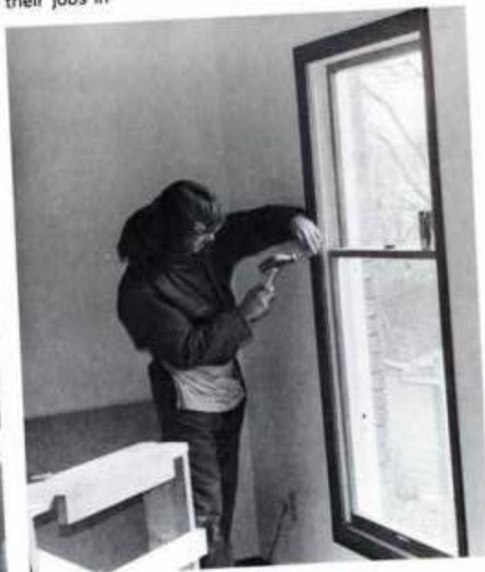
Kenny Green takes aim at a window frame for a new condominium as part of his work as a carpenter's helper, through the ICT program, for Phillips Construction.
