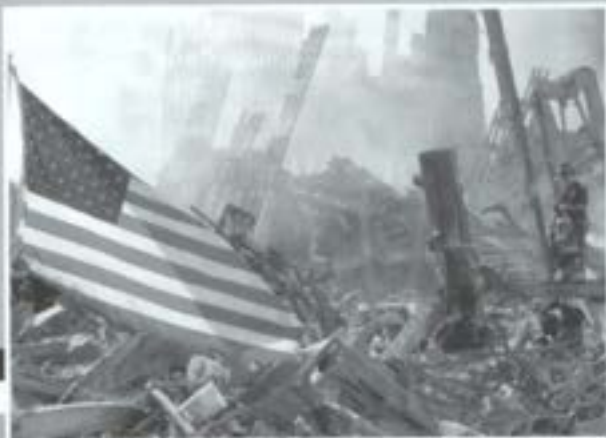
New York City, NY, September 16, 2001-FEMA Urban Search and Rescue teams work to clear rubble and search for survivors at the World Trade Center. (Photo by Michael Rieger/FEMA News Photo)
